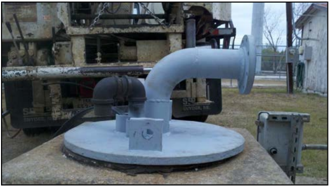
New Wellhead with 4" pipe at well #14
