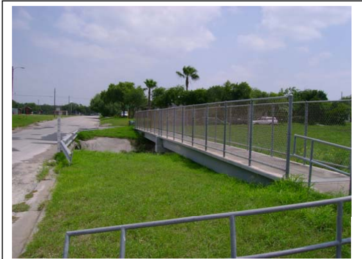
There are several pedestrian bridges crossing over the creek in the north part of Kingsville. These bridges help enhance pedestrian connectivity between neighborhoods and to destinations in the community. Several of the bridges do not currently connect to sidewalks and an opportunity exists for the City to connect these bridges through sidewalk construction and/or through developing a trail system along the creek.
