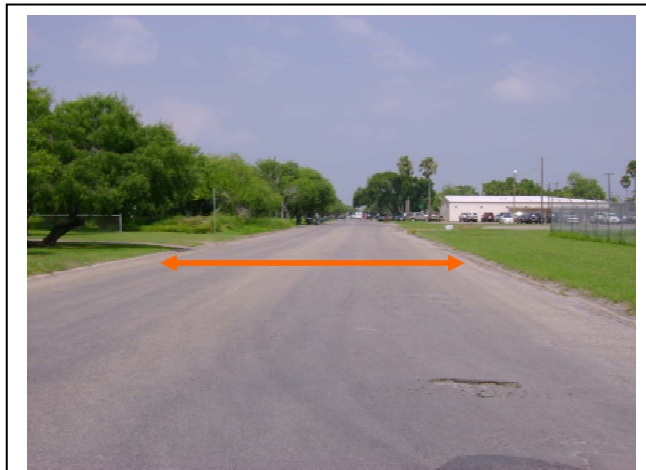
Many of the roadways are wide in Kingsville and could easily accommodate amenities including bike lanes or on-street parking.
