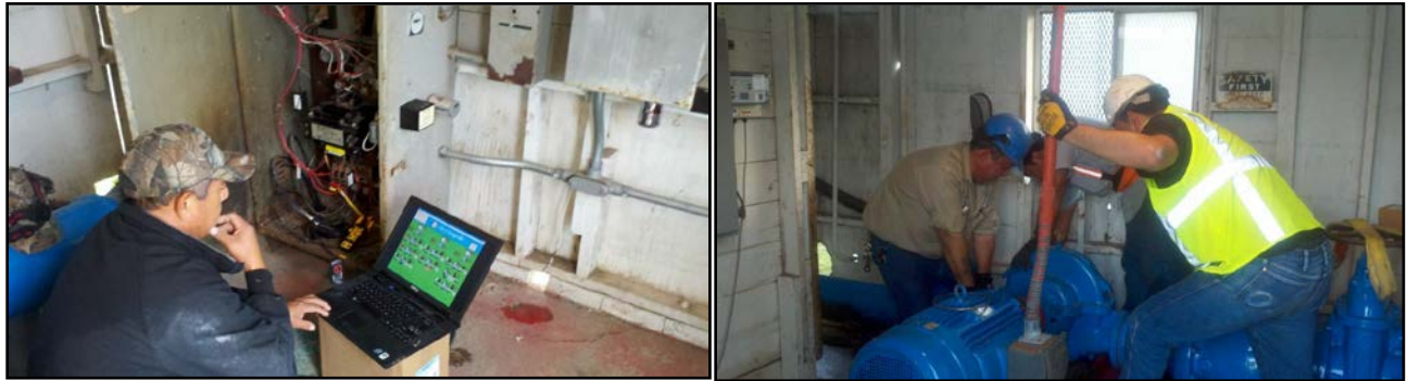
Field Calibration of the SCADA System by Water Production supervisor Water production Crews are installing booster pump at Well #17
