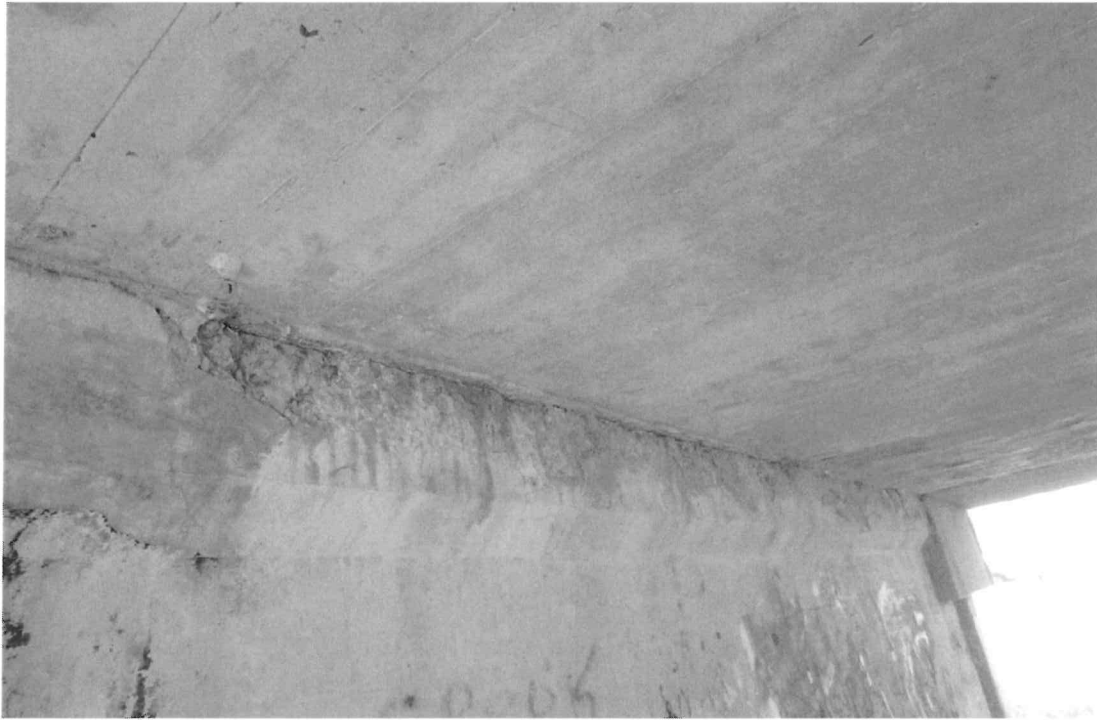
VIEW 9 - MINOR DELAMINATION & SPALLING ALONG TOP EDGES (BEARING AREAS) OF ORIGINAL PIER WALLS & WIDENED CAP BEAMS AT THE 2 SOUTH BENTS.
