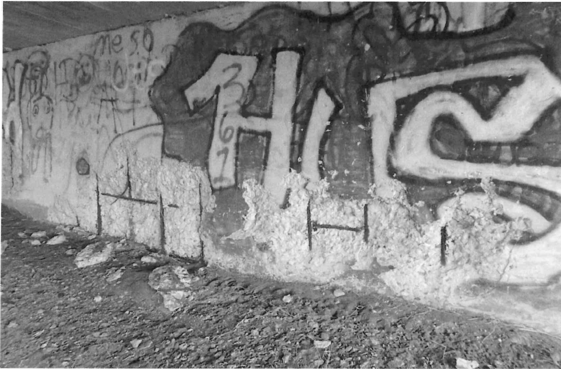
VIEW 7 - SEVERAL MODERATE SPALL WITH EXPOSED REBAR IN SOUTH ABUTMENT WALL
