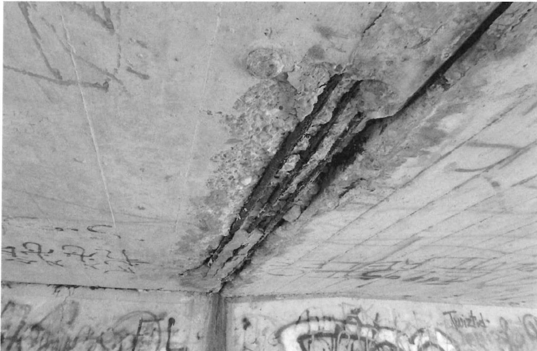
VIEW 8 - HEAVY SPALL WITH EXPOSED REBAR IN SOFFIT OF SLAB IN NORTH SPAN ALONG CENTER WIDENING JOINT.
