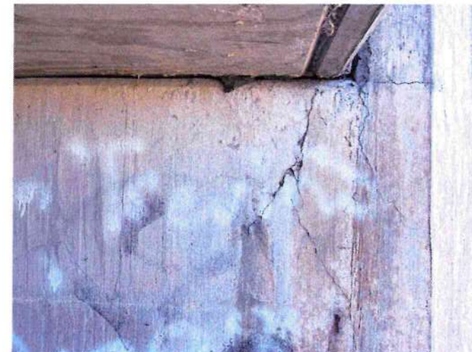
6 C20 NTS TYPICAL CRACK AND SPALLING OF CONCRETE
