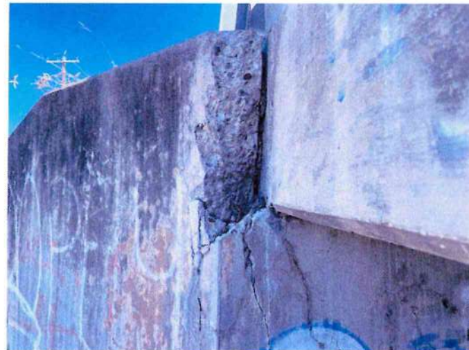
5 C20 NTS TYPICAL CRACK AND SPALLING OF CONCRETE
