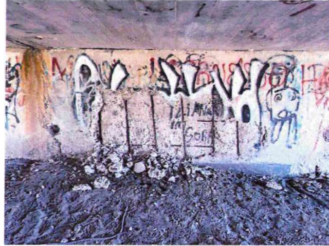
1 C20 NTS TYPICAL CONCRETE SPALL WITH EXPOSED REBAR
