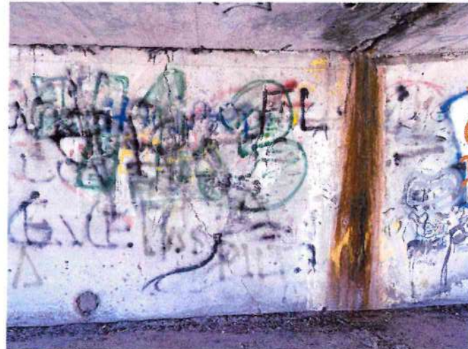
4 C20 NTS TYPICAL CRACK AND SPALLING OF CONCRETE
