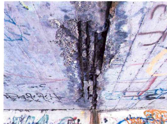
3 C20 NTS TYPICAL CONCRETE SPALL WITH EXPOSED REBAR
