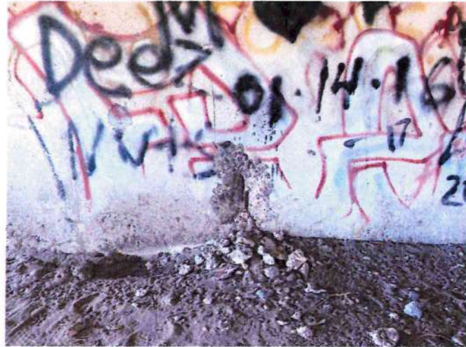
2 C20 NTS TYPICAL CONCRETE SPALL WITH EXPOSED REBAR
