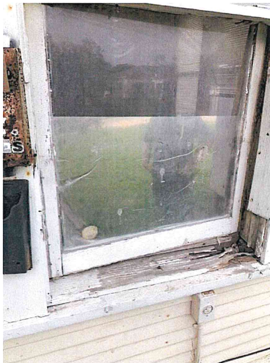
Windows-Damaged beyond reasonable repair
