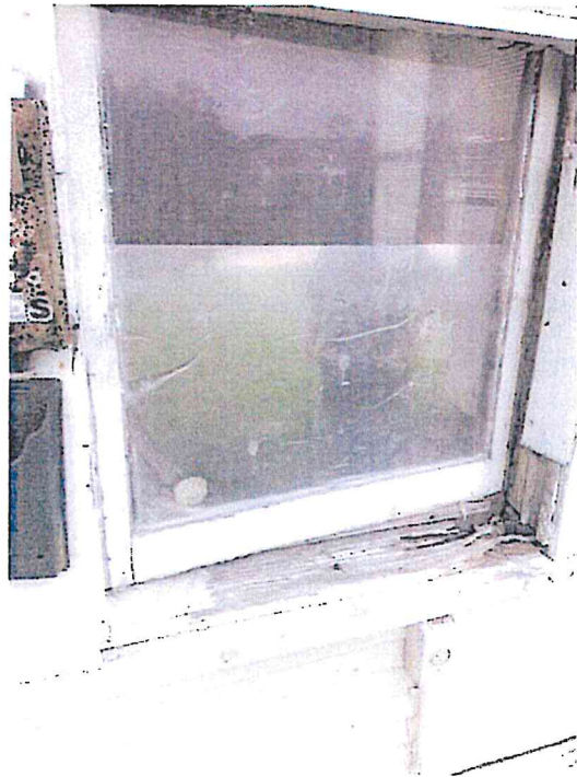
Windows-Damaged beyond reasonable repair
