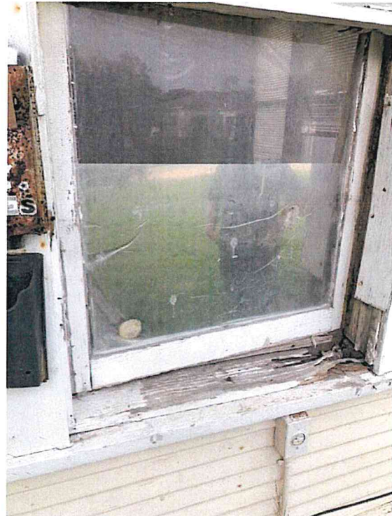
Windows-Damaged beyond reasonable repair
