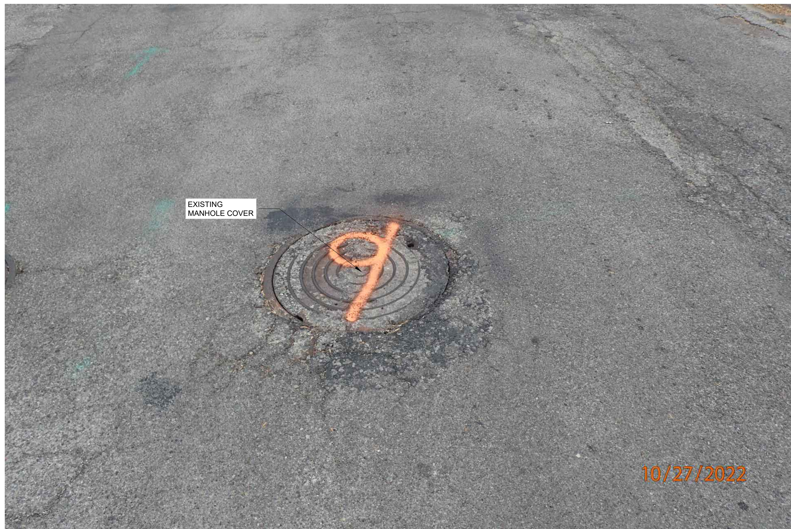
1 SANITARY SEWER MANHOLE 9 EXISTING EXTERIOR REHABILITATION PLAN (PHOTO) C12 C12 SCALE: N.T.S.
