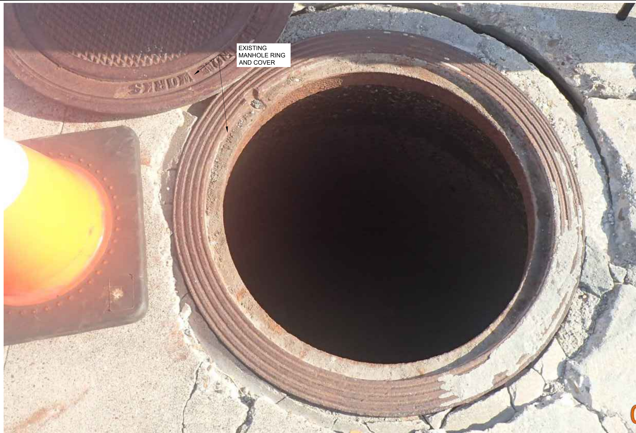
1 SANITARY SEWER MANHOLE 11 EXISTING EXTERIOR REHABILITATION PLAN (PHOTO) C14 C14 SCALE: N.T.S.
