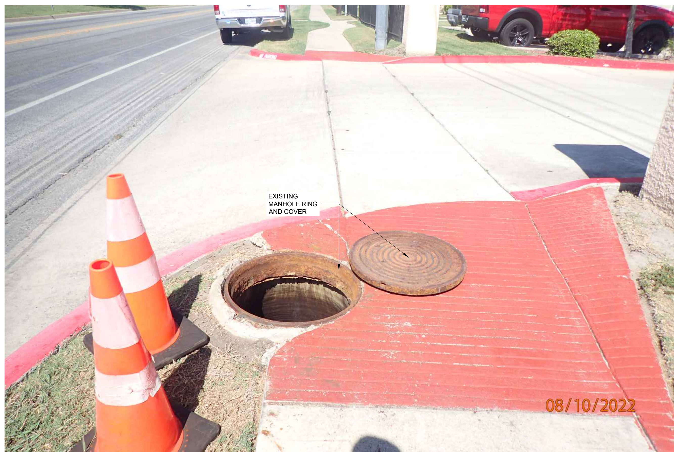
1 SANITARY SEWER MANHOLE 10 EXISTING EXTERIOR REHABILITATION PLAN (PHOTO) C13 C13 SCALE: N.T.S.
