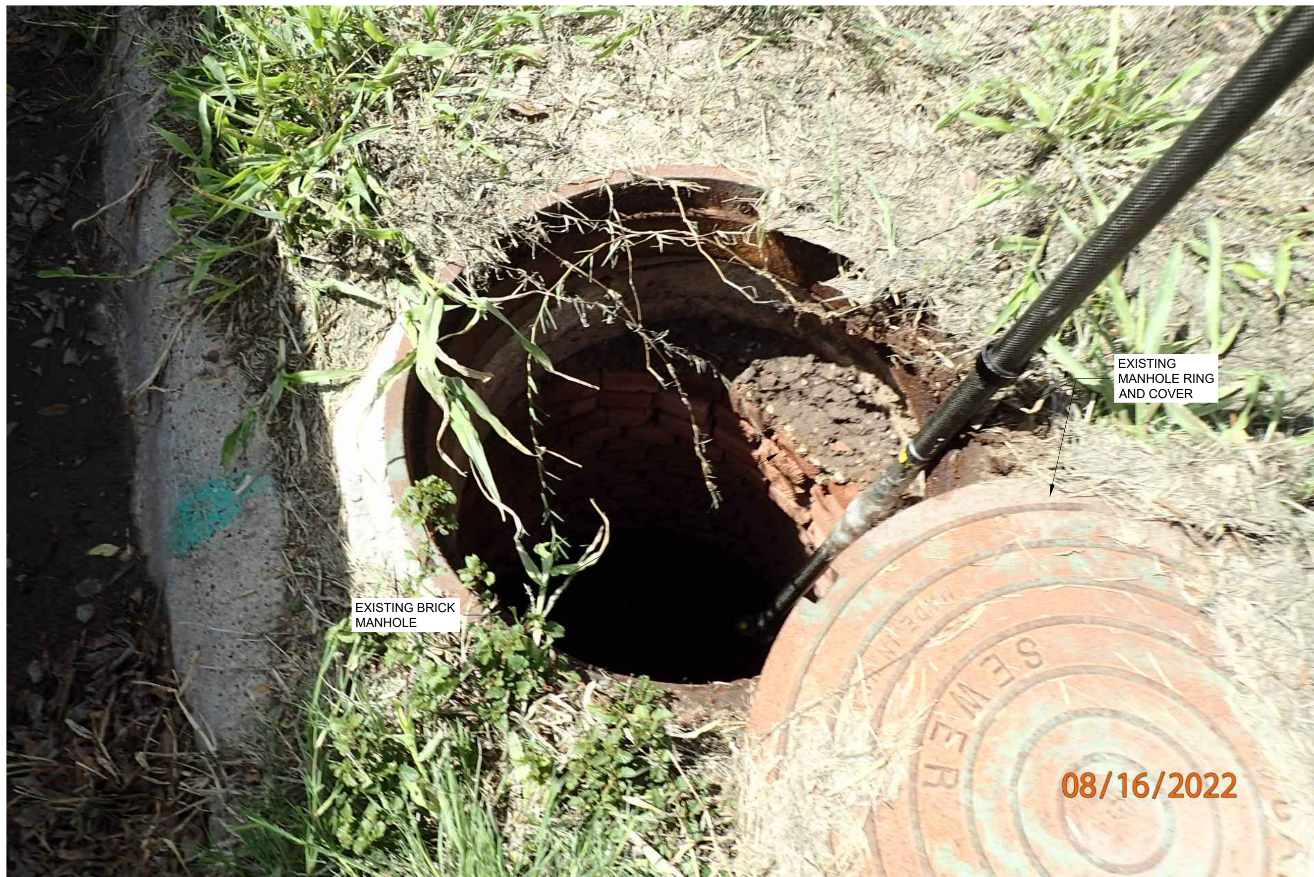
1 SANITARY SEWER MANHOLE 30 EXISTING EXTERIOR REHABILITATION PLAN (PHOTO) C30 C30 SCALE: N.T.S.
