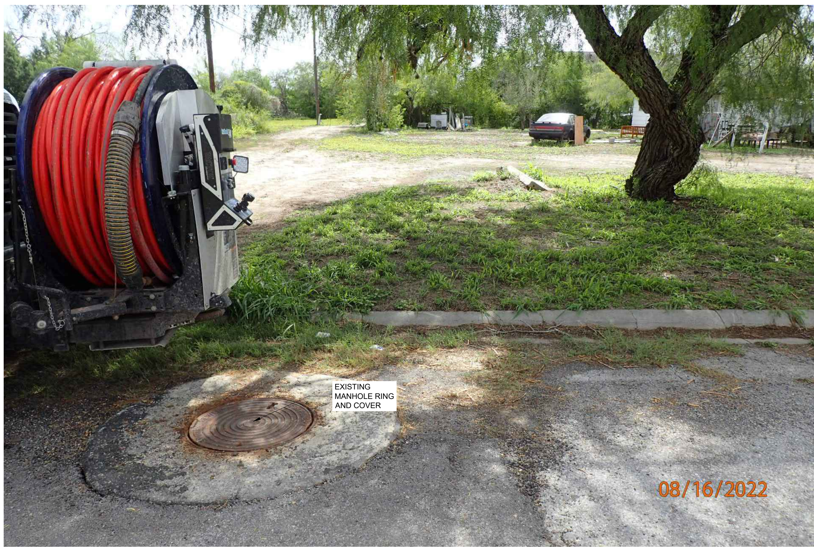
1 SANITARY SEWER MANHOLE 28 EXISTING EXTERIOR REHABILITATION PLAN (PHOTO) C28 C28 SCALE: N.T.S.
