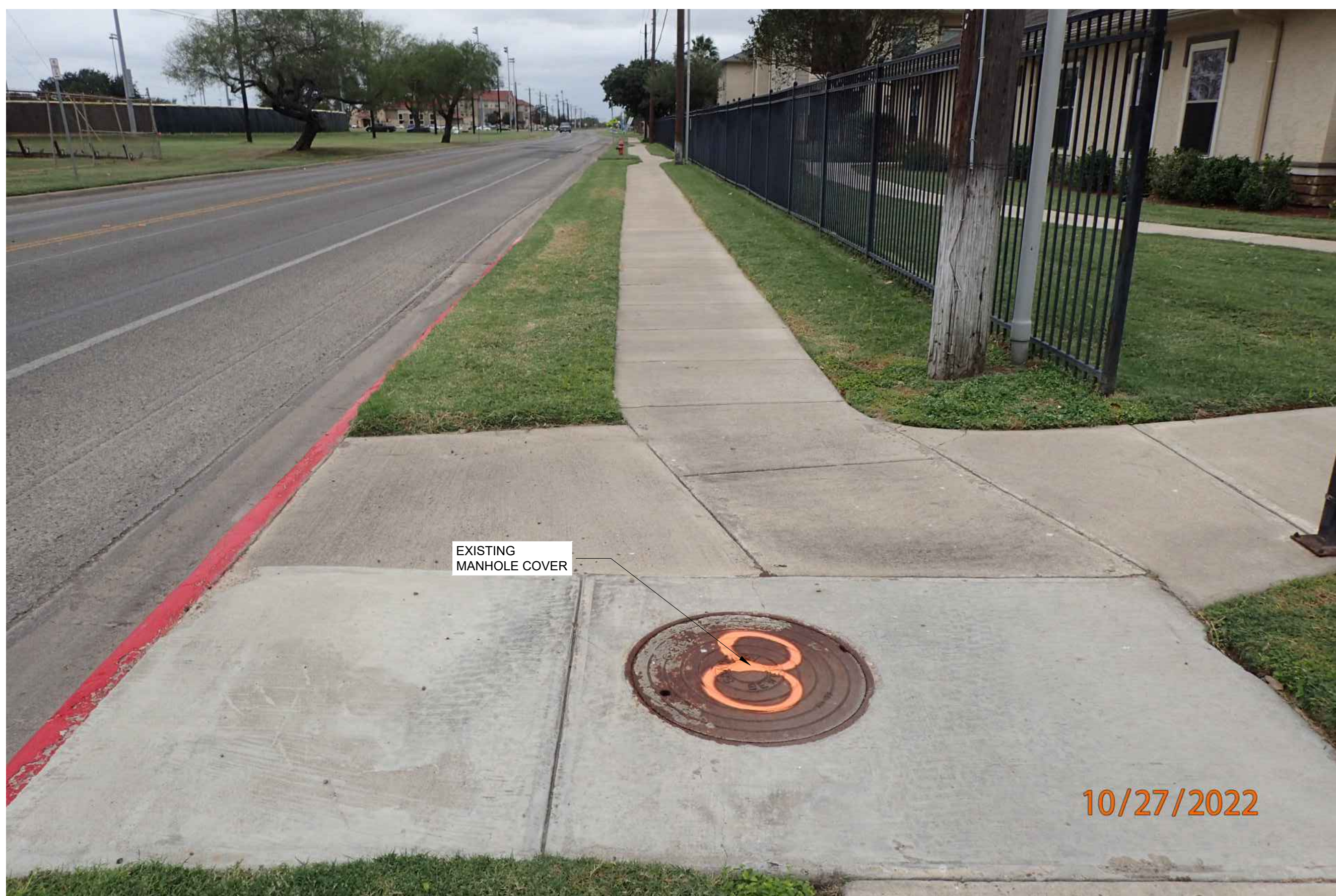
1 SANITARY SEWER MANHOLE 8 EXISTING EXTERIOR REHABILITATION PLAN (PHOTO) C11 C11 SCALE: N.T.S.
